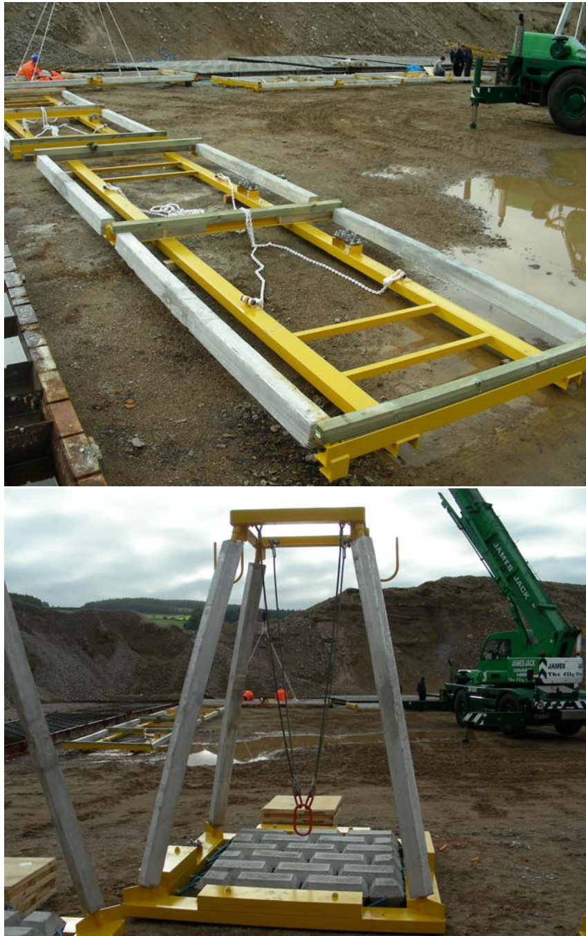
FIGURE 2 EXAMPLES OF ANODE RETROFIT SLEDS AND PODS USED IN THE FORTIES INFIELD PIPELINES ANODE RETROFIT PROGRAM
